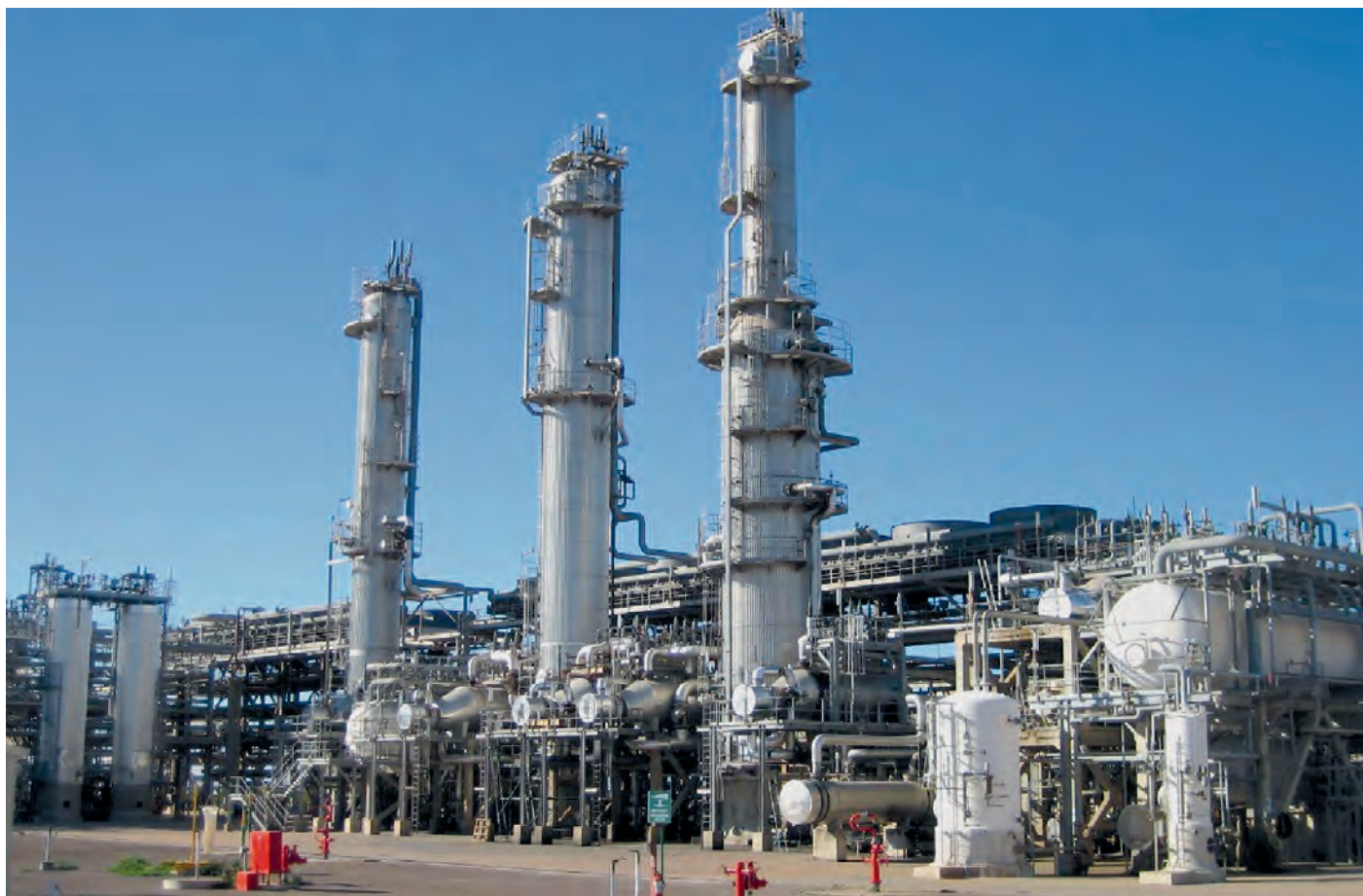
The LPG fractionation columns at Port Bonython.
