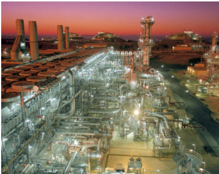
One of the LNG Production Trains at the Karratha Gas Plant
