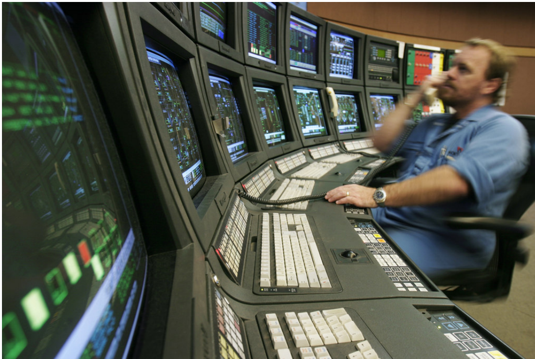
Central Control Room operations of the Condensate Stabiliser Units
